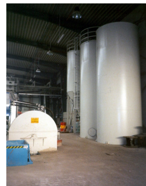
FLOTMAT with AQUACLEAN and clear water silos.
